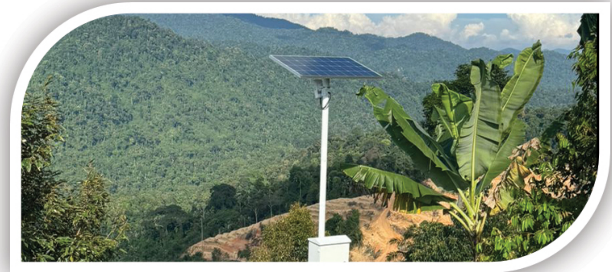
Solar CCTV for Estate
